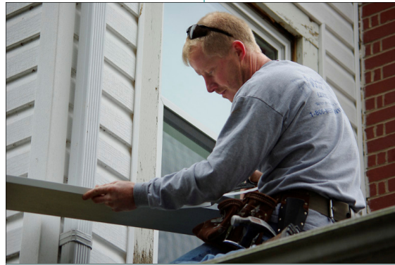
Window World's Ken Rhodes puts the finishing touches on one of the 28 new windows that were installed at SAFE's shelter recently. The windows were a gift from Window World. Upgrades to the shelter's HVAC, plumbing and electrical systems will start soon, with security enhancements and outdoor improvements to follow in the spring.
